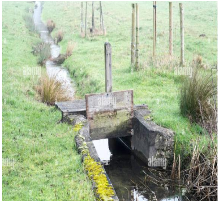
wooden sluice gate
