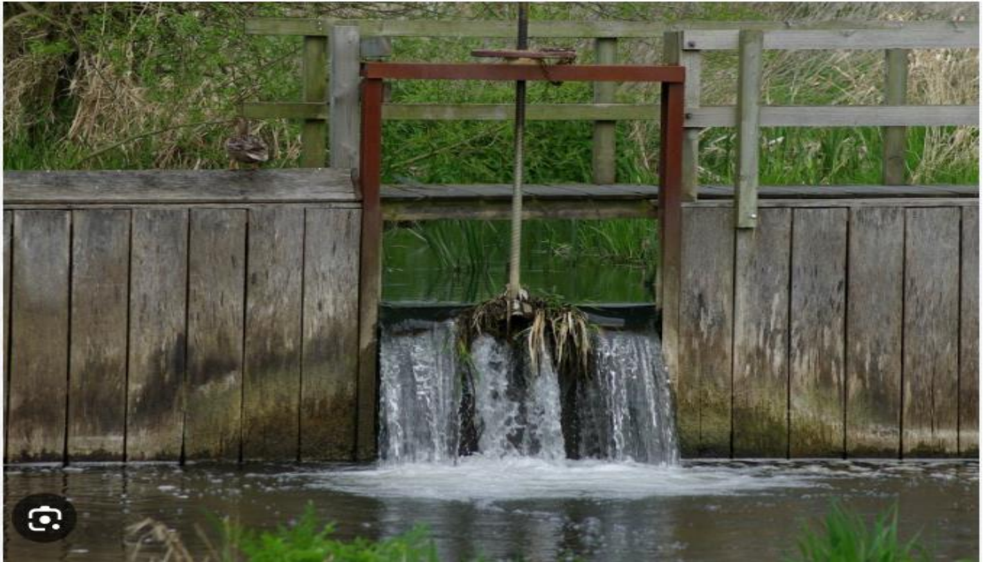
Sluice gate control
